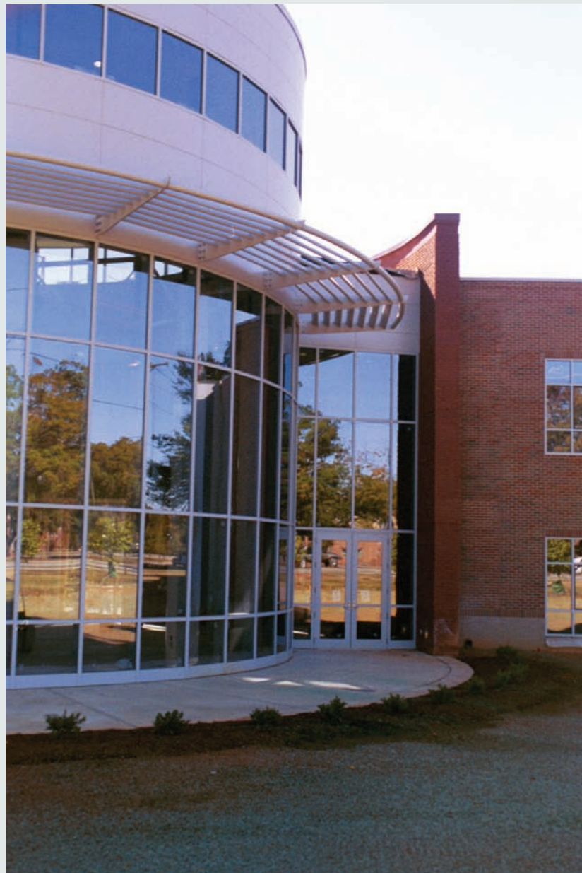
The architect incorporated a shading device on the north-facing façade of this building. As a result, the expensive shading lattice provides no shading benefits and adds over $10/ft 2 to the total building cost. On the same building, the east-facing windows are completely unprotected.
